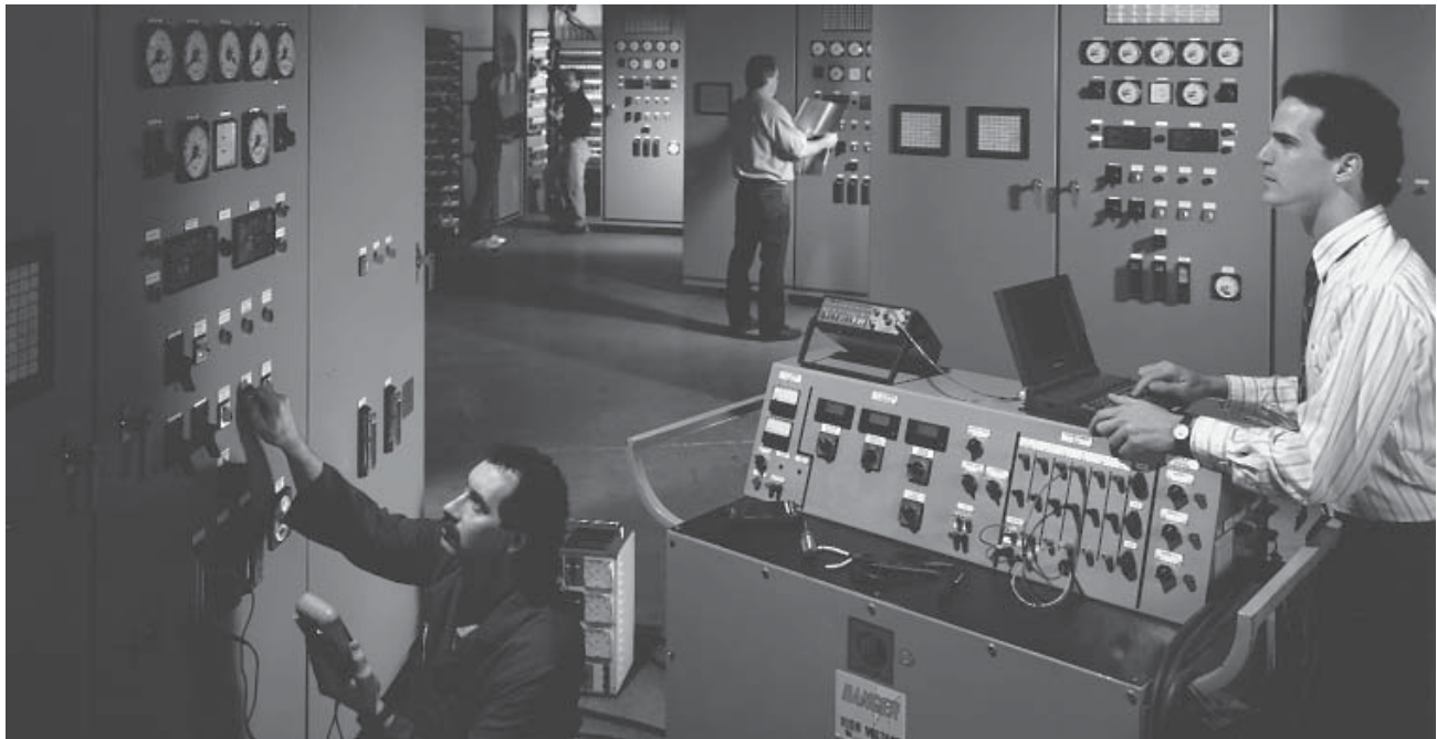
17.6MW Series System Control for Cernavoda Nuclear Power Plant, Romania
